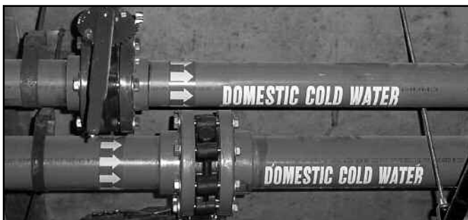
Butterfly valves installed with Corzan pipe.
