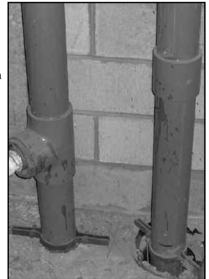
Typical riser supports using Corzan pipe.
