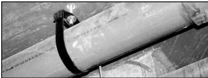
Typical pipe hangers.
